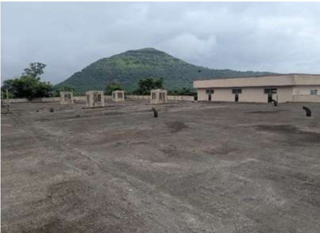
Figure 30 Clear Water Tank
